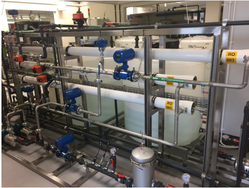
Figure 2: The Secure Water Treatment (SWaT) testbed
